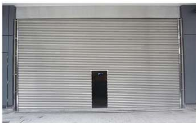
Stainless Steel Shutter at CLP's Station at Shatin Wales of Prince Hospital
